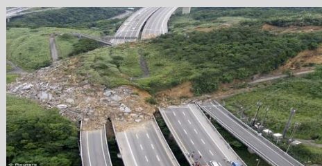
Figure 1: Slope failure on motorway No. 3 of Taiwan.
