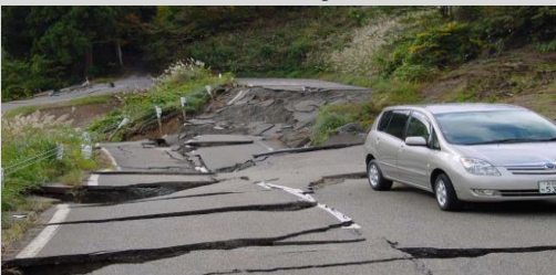
Figure 3: Road damage during the Niigata - Ken Chuetsu earthquake (Japan)
