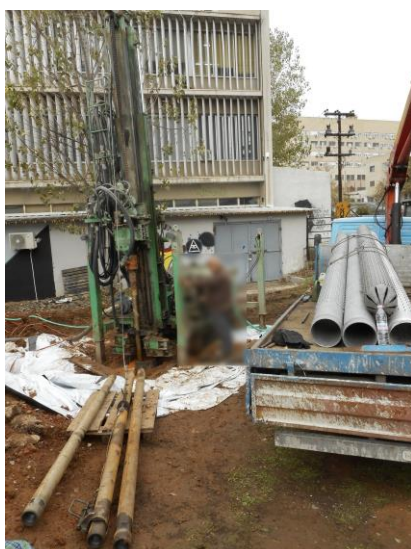
Figure 3. A moment of the construction process, by the Hydraulics Lab, Aristotle University of Thessaloniki.
