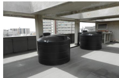
Figure 4. The water tanks properly placed on the roof of the building.
